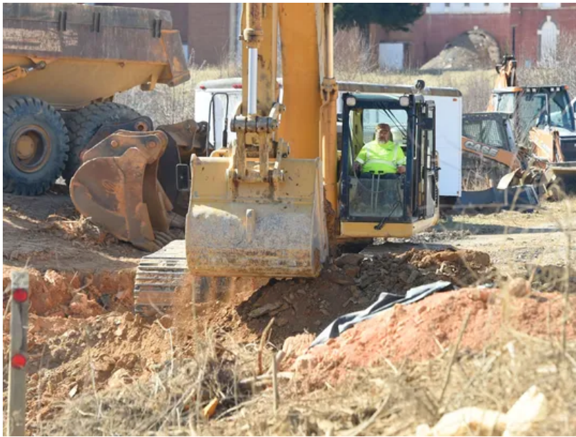
An excavator works to move earth and load dump trucks. Construction continues on land designated for the Frontier Center project, alongside the road that leads to the entrance of the Frontier Culture Museum in Staunton on Monday, Feb. 20, 2017. (Photo: Mike Tripp/The News Leader)
